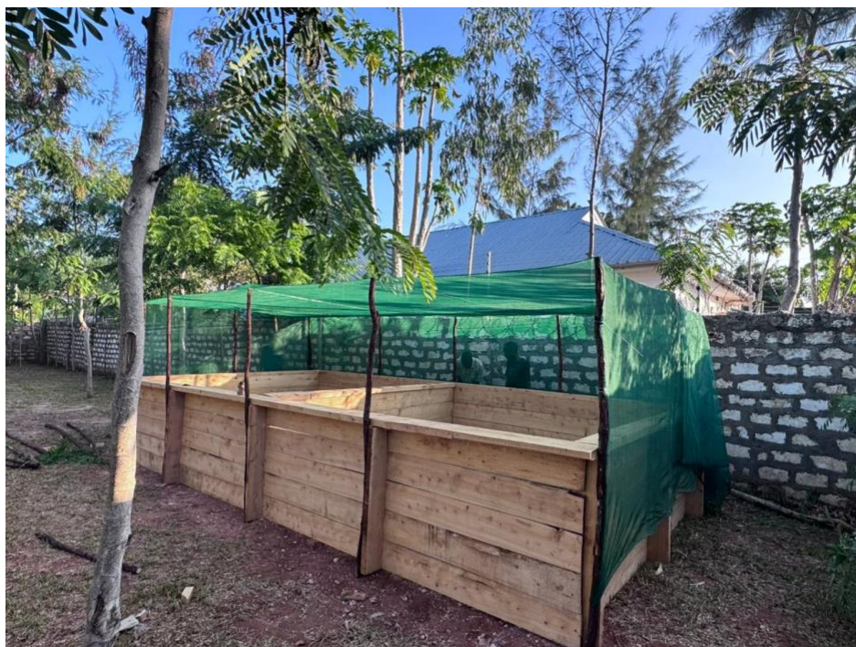
Figure 3: the newly constructed wooden ponds to be used as broodstock ponds. the ponds will be lined with a pond liner to ensure water retention.
